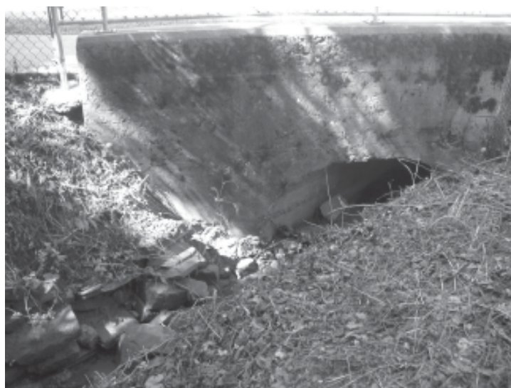
Constriction points created by older railroad or automobile bridges can cause local flooding.
