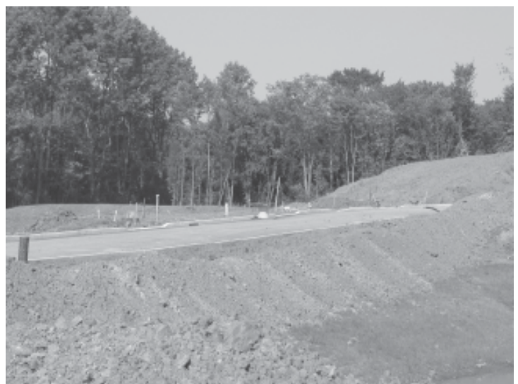
Construction sites, if not managed well, can be major contributors to polluted stormwater runoff.
