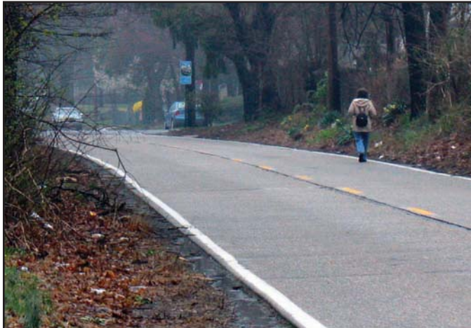
Segments of the corridor lack sidewalks. Coupled with narrow shoulders and sloping berms along the roadside, pedestrians are often forced to walk in the cartway. Source: DVRPC
