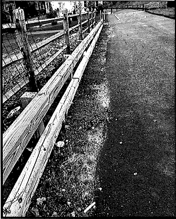
Item #16 – Emergney Access Drive edges in disrepair
